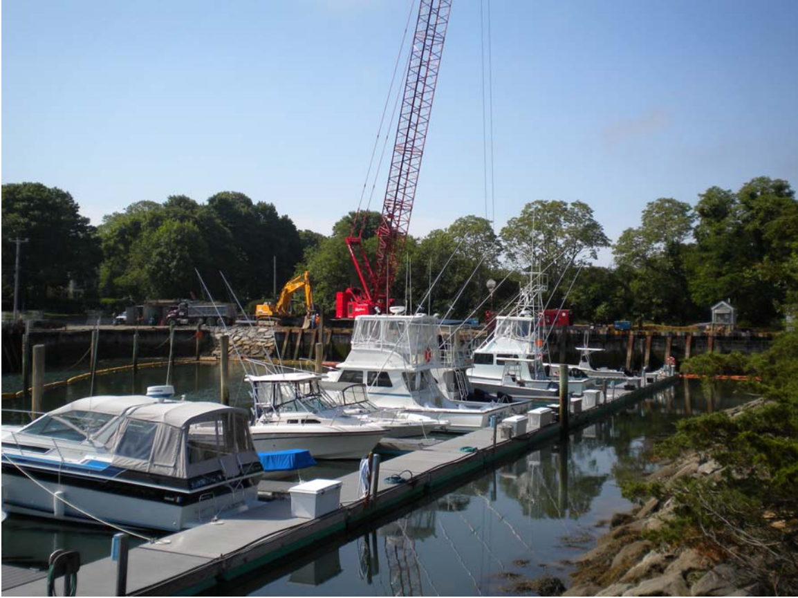
Construction on the new bulkhead at the Barnstable Harbor Marina. Seventy-five percent of this $5 million project is being paid for with a state grant. The anticipated completion date for the project is November 2010.
